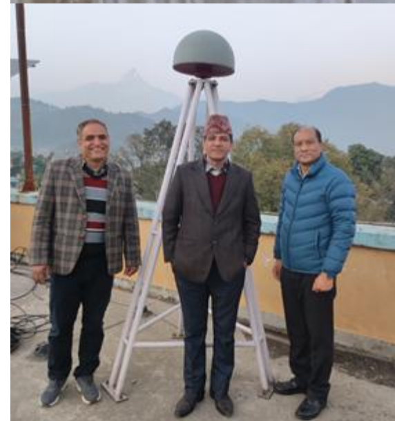
Construction of Bench Mark for GNSS Training Purpose: Compare GNSS accuracy based on various processing techniques such as SPP, DGPS, SBAS, RTK, PPK, MADOCA PPP, PPP etc.
